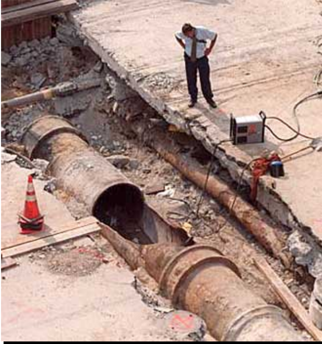
Figure B-9. An official surveys the gaping hole in a broken 40-inch water main at Howard and Lombard streets in Baltimore, Maryland.
